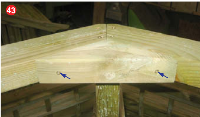
Using 2 x 40mm screws, secure a corner support in each corner of the top frame.
